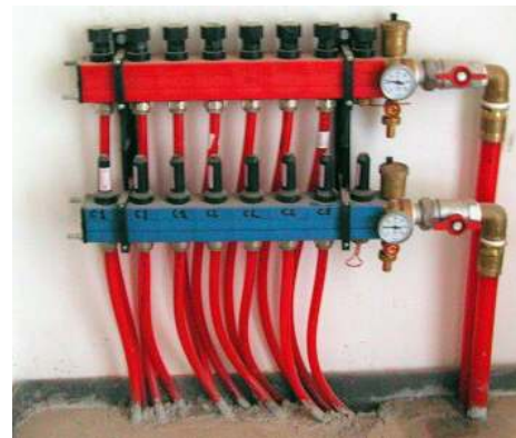
PEX piping. Photo: Chixoy
